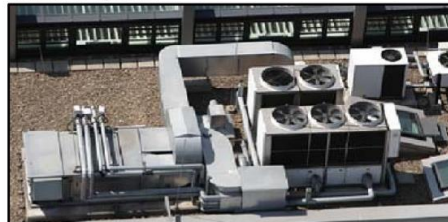
Chiller AC system
